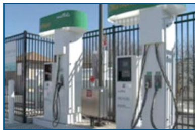
Hydrogen fueling station in Hempstead, Long Island
