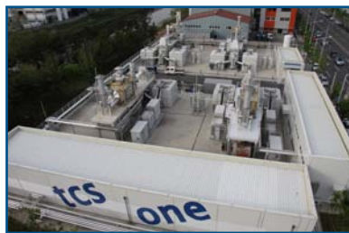
Four 2.8 MW FuelCell Energy power plants providing clean power to the South Korean electric grid
