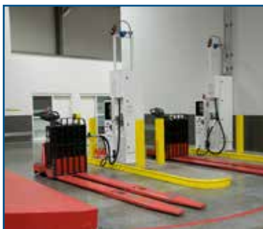
Indoor fueling of a material handling pallet jack. Photo courtesy of Air Products and Chemicals, Inc.
