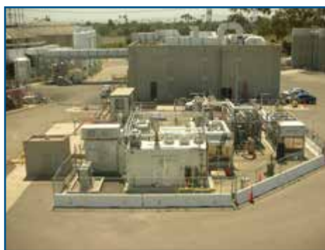
OCS Energy Park producing heat, power, and hydrogen from anaerobic digester gas. Photo courtesy of Air Products and Chemicals, Inc.
