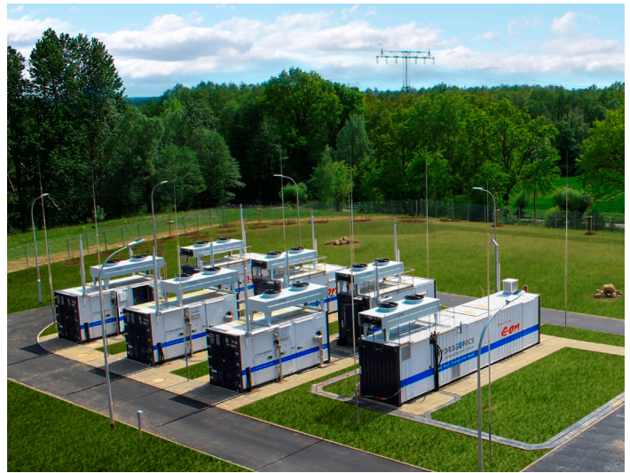
Figure 5. Hydrogenics P2G facility in Falkenhagen, Germany. Photo courtesy of Hydrogenics.
