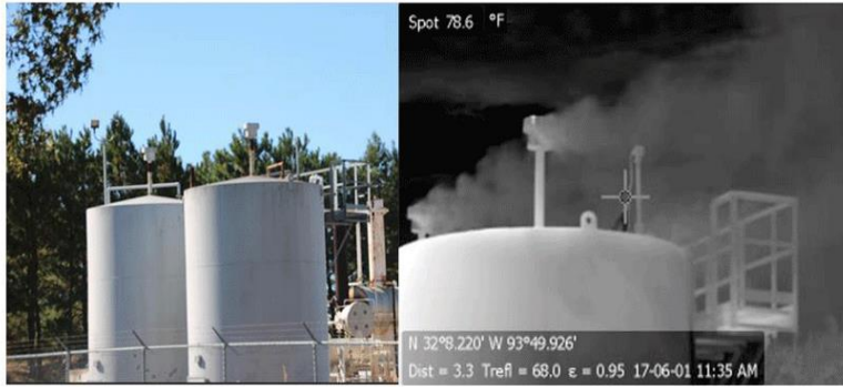
Figure 2. Natural gas storage tanks at the Haynesville, Texas, shale fields. Picture on left taken with a normal camera. Picture on right was taken with forward-looking infrared (FLIR) camera tuned to the infrared spectrum of methane, which allows visualization of methane emissions. Photo courtesy of Sharon Wilson. Reprinted from Howarth (2019). 3
