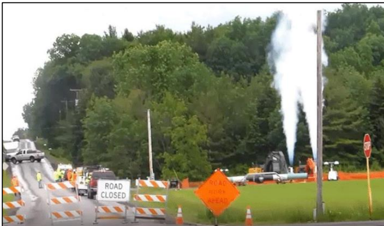
Figure 3. Blowdown for maintenance of a natural gas pipeline in Yates County, New York. Methane is an invisible gas, but the cooling from the rapid blowdown condenses water vapor, leading to the obvious cloud. Photo courtesy of Jack Ossont. Reprinted from Howarth (2019). 3
