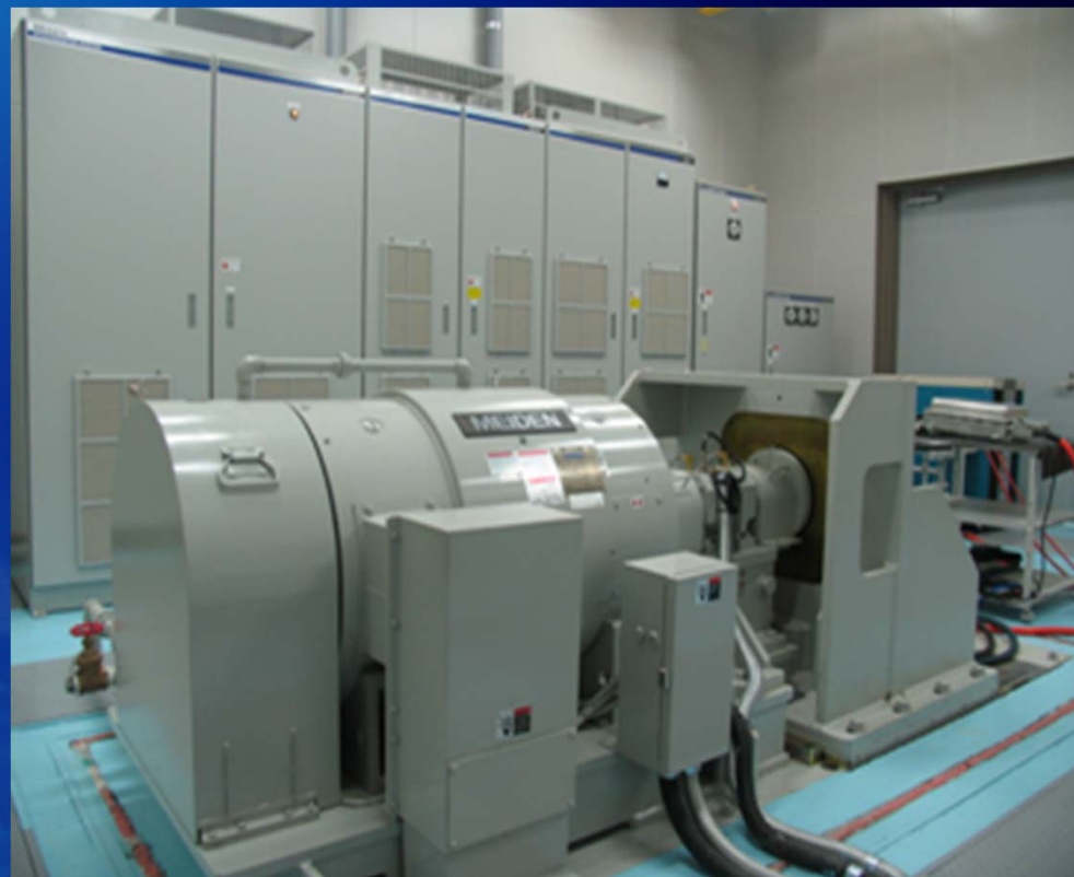
Motor Test Equipment (250 kW Class)
