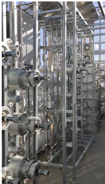
Gas Management Panels
