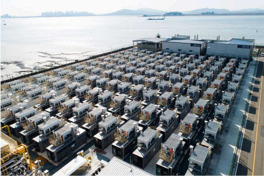
Western Incheon Fuel Cell Power Plant, S. Korea, where Doosan Fuel Cell's 58.96 MW are installed (440kW PAFC modules)
