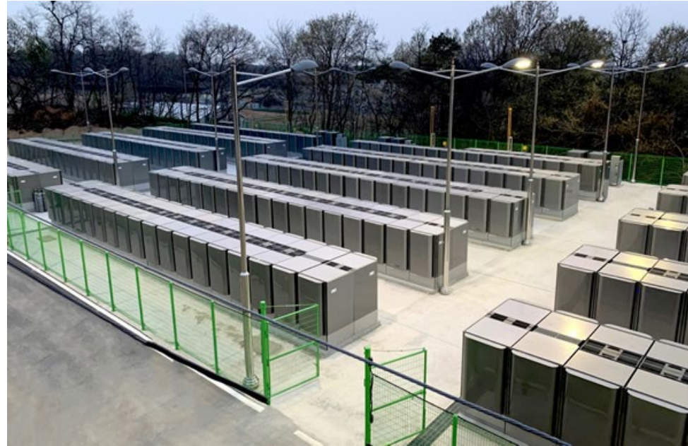
Bloom Energy 19.8 MW fuel cell deployment of Bloom Energy Servers, Hwasun, S. Korea (200kW SOFC modules)
