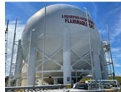
LH 2 storage tank 5,000 m 3
