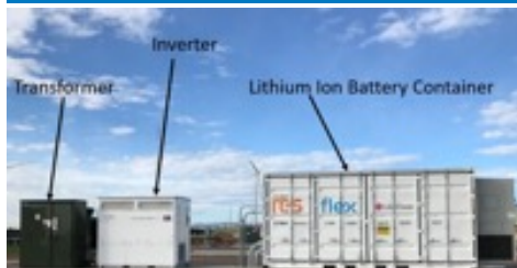
Battery 1MW / 1MWh
