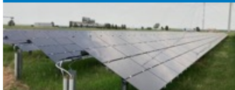
Solar PV with Inverter Controls
