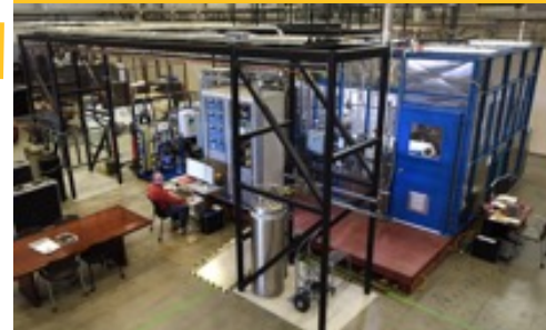
High Temp Electrolyzer
