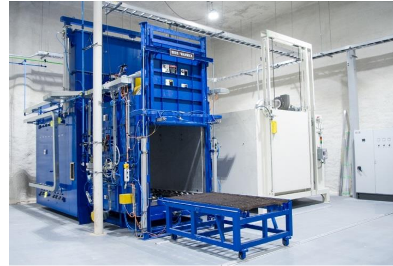
Mainstream's CAB furnace facility
