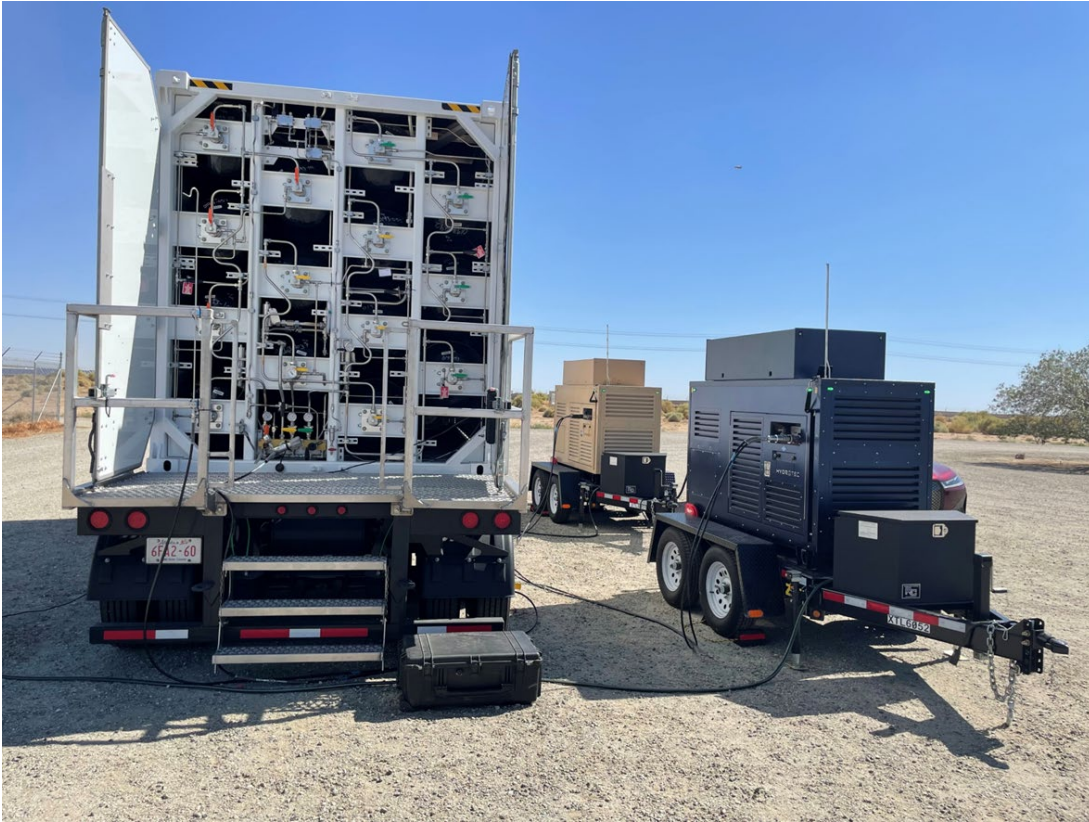
MPGS (Mobile Power Generation System) setup in the field as part of Hydrogen Ecosystem Project
