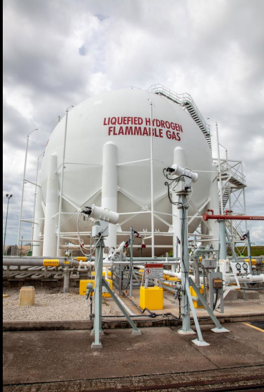
LH2 Tank at Pad 39B
