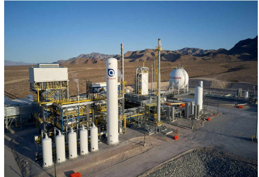
Air Liquide's North Las Vegas Hydrogen Liquefaction Plant
