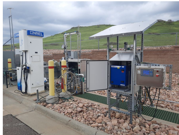
Integration of an HCD at the NREL Dispenser The HCD enclosure regulates environmental parameters for HCD operation and is positioned outside the electrically classified area to facilitate deployment.
