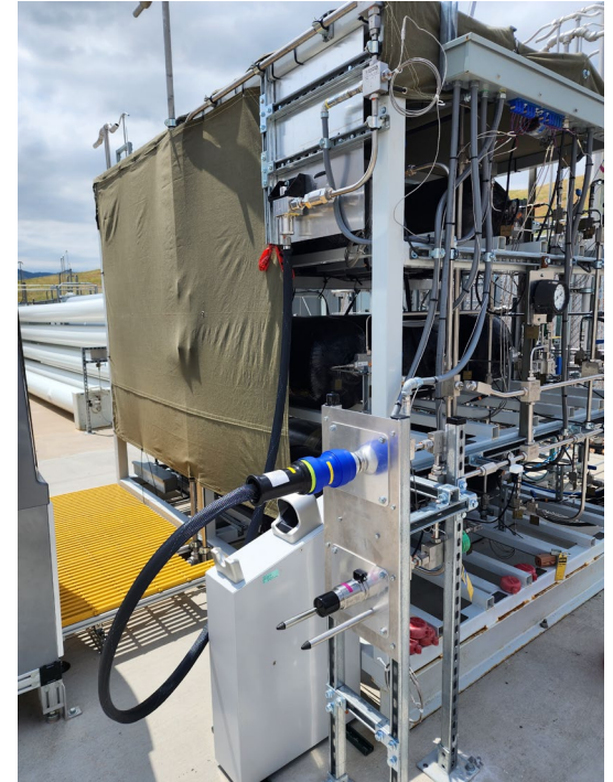
Industry Provided Hardware Installed at NREL's Heavy-Duty Hydrogen Fast-Flow Research Facility
