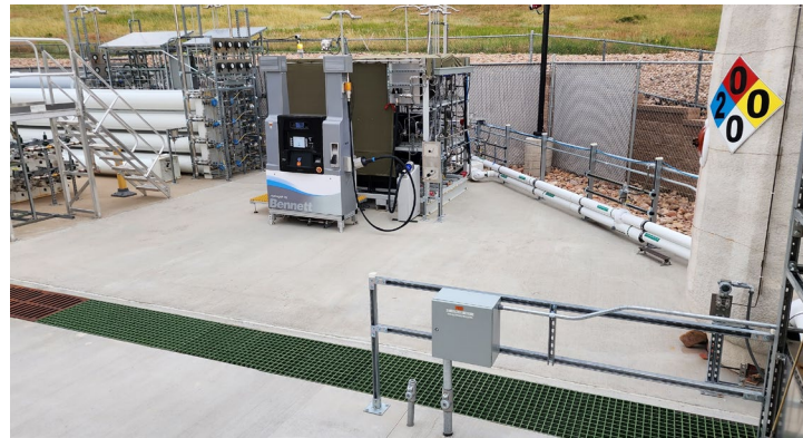
NREL's Heavy-Duty Hydrogen Fast-Flow Research Facility
