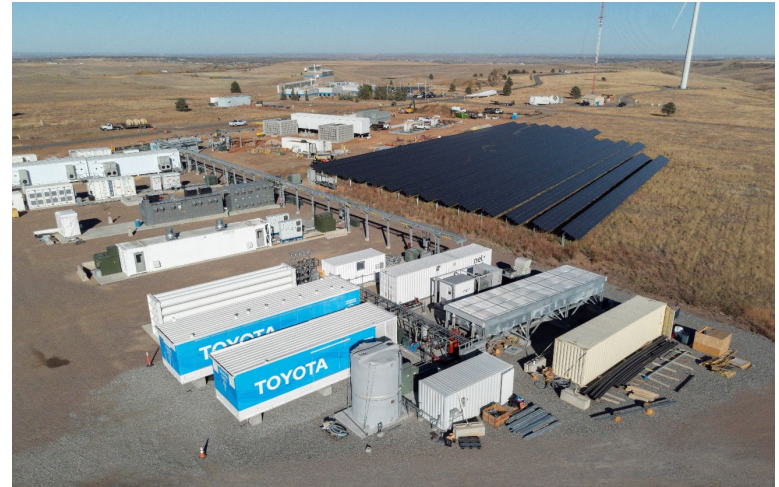
Hydrogen system at ARIES. Photo by NREL
